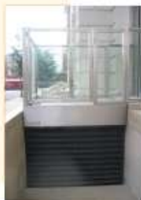
Disabled access lift with bellows protection
